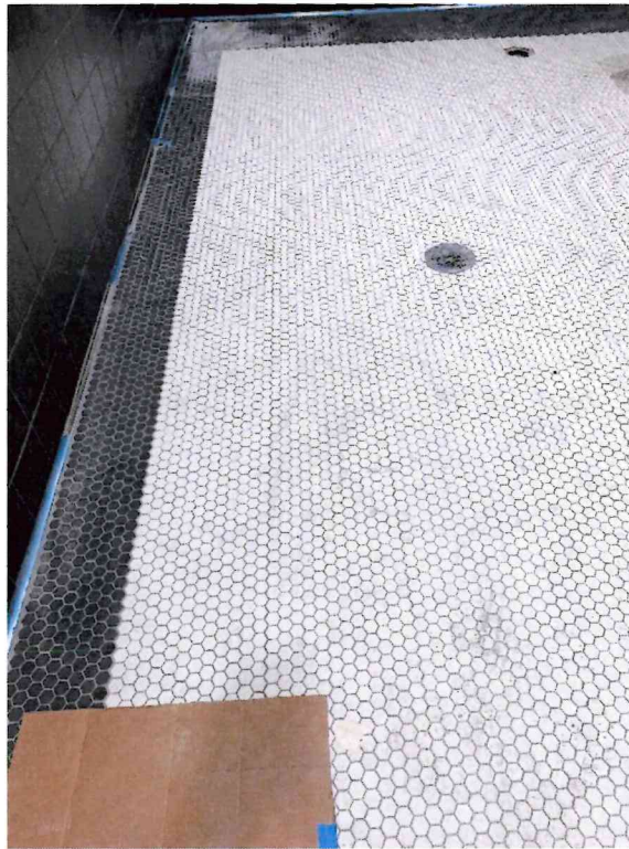
Floor Tile Grout Line Defects
